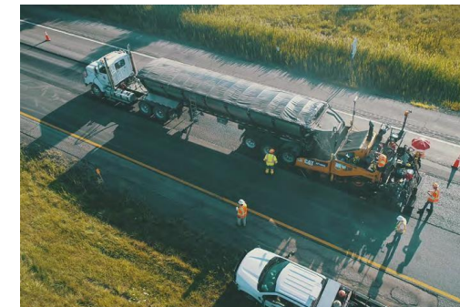
Recycled asphalt pavements RAP/ micro-milling technique, on the route 81 in the State of New-York, in the USA
